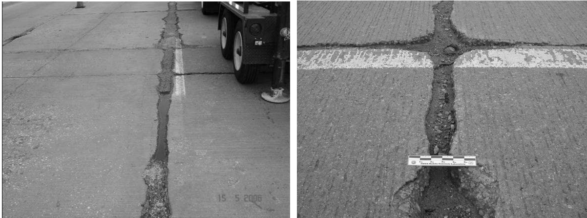
Fig. 1. Section of pavement on W 86 th Street, Indianapolis, IN (left) and SR 933 near South Bend, IN (right)
