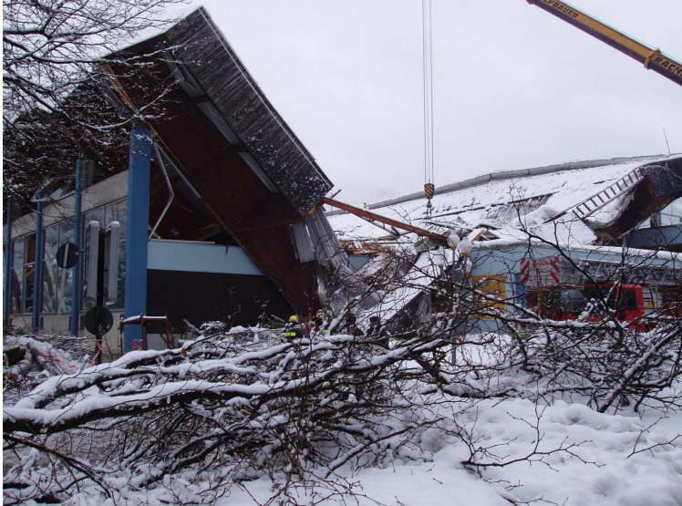
Fig. 1: Collapsed ice stadium (January 2006)
