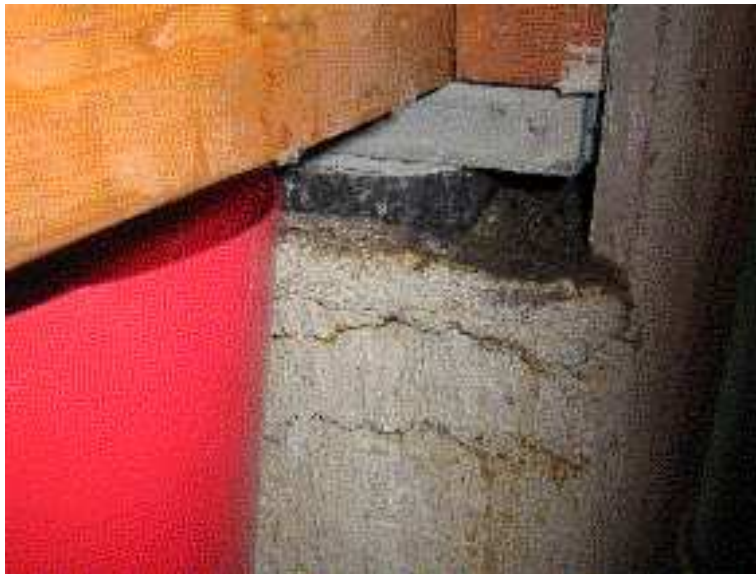
Fig. 10: ... resulting in corrosion of the bearing
