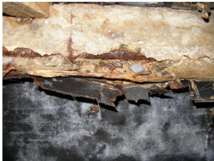
Fig. 16: Water penetration into isolating material
