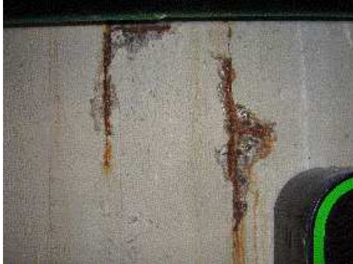
Fig. 13: Corrosion of ferro-concrete due to insufficient covering
