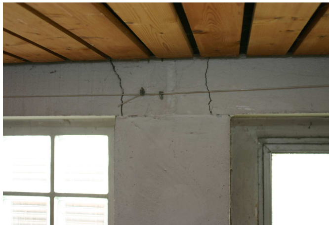
Fig. 6: Concrete structure with insufficient shear resistance
