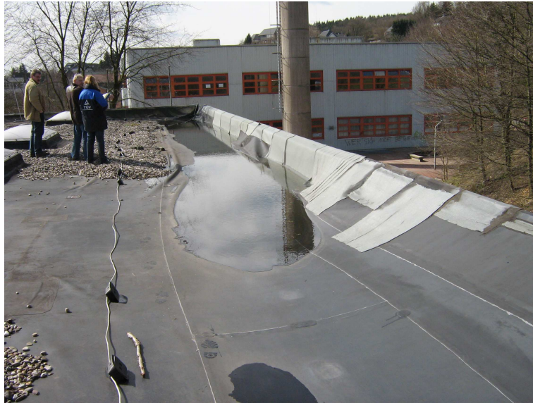
Fig. 9: Bad repair of roof coating
