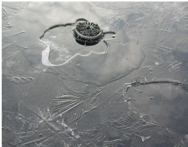
Fig. 8: Wrong position of a sink on a flat roof
