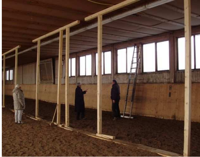
Fig. 4: Ceiling on wooden window frames
