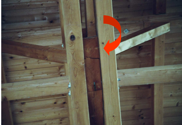
Fig. 7: Insufficient distance of bore holes
