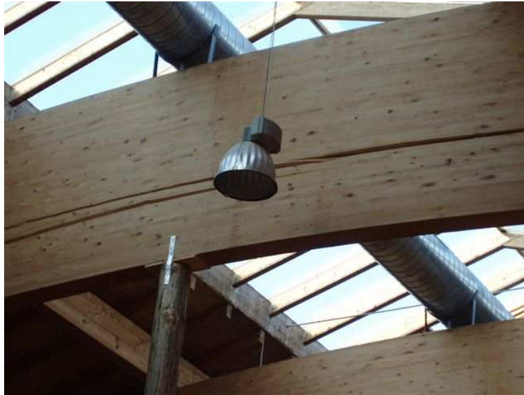
Fig. 11: Wooden truss divided by a penetrating fissure
