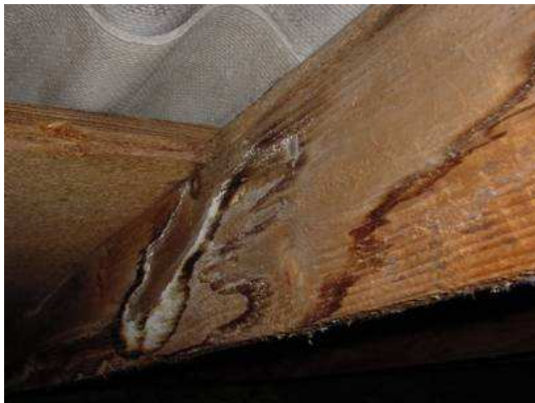
Fig. 12: Wooden truss affected by humidity
