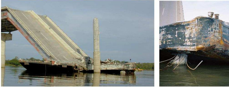
Fig. 4. Views of Damage at Webber Falls (Courtesy of Zolan Prucz)
