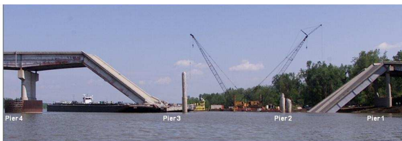
Fig. 3. Views of Damage at Webber Falls (Courtesy of Zolan Prucz)
