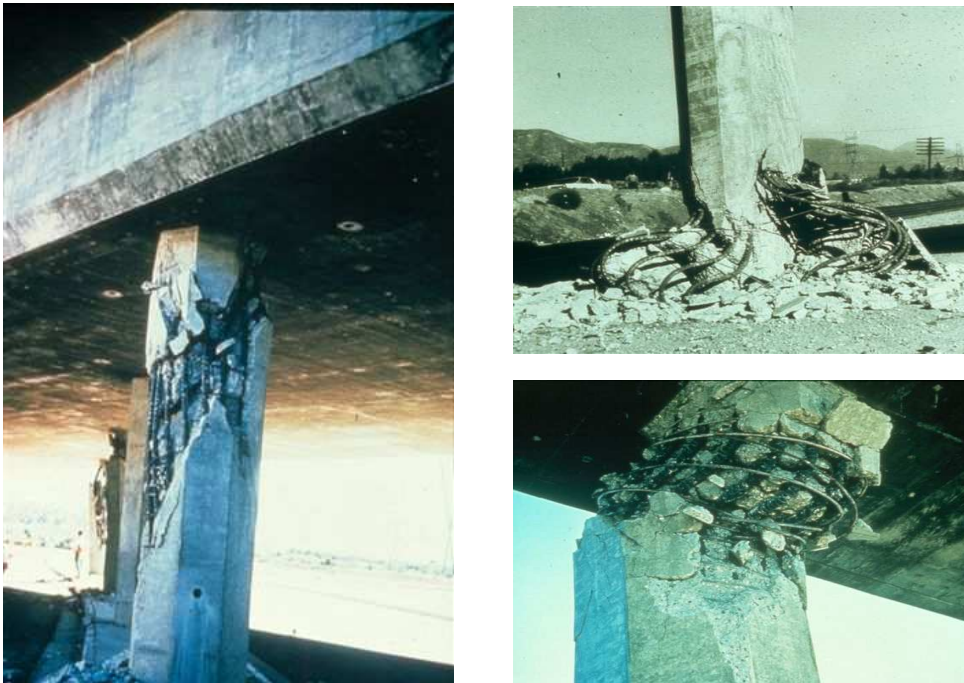
Fig. 17. Typical Column Damage from 1971 San Fernando Earthquake (Source: California DOT Photo Archives)
