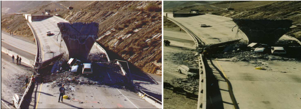
Fig. 19. Damage from 1994 Northridge Earthquake (Source: University of Buffalo/MCEER Photo Archives)
