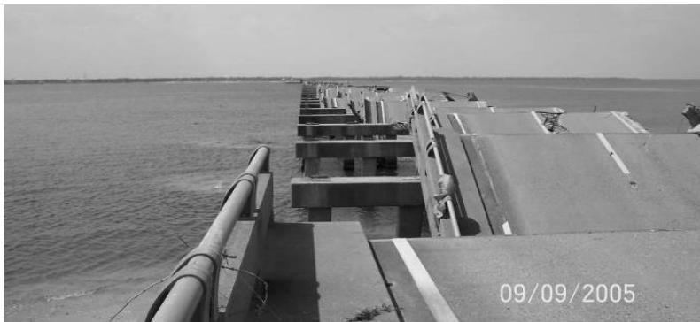
Fig. 20. Dislodge Spans of US 90 Bridge over Bay St. Louis, Mississippi, Resulting from Hurricane Katrina 2005 (Courtesy of Mississippi DOT)
