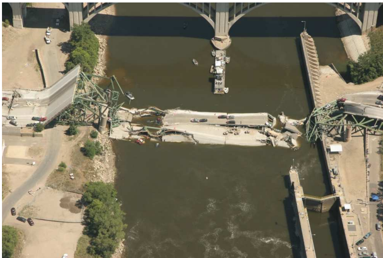
Fig. 22. Aerial View of Collapsed I-35 W Bridge, Minneapolis, Minnesota (Courtesy of FHWA)
