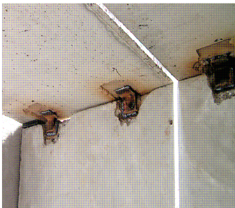
Fig. 6. Connection vulnerable to Fire
