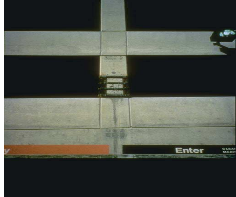
Fig. 10. Short Column failure – Northridge earthquake (1995) – Parapet walls reduced the height of columns
