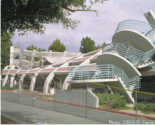
Fig. 9. Parking garage – Northridge earthquake (1994) – inadequate capacity of non participating elements
